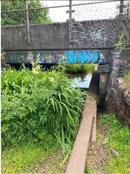
Plate 9: The Site as it passes below the Glasgow-Helensburgh railway. Note flooding beneath the bridge structure.
